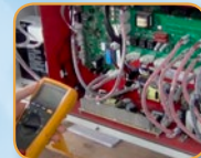
Checking the Electrical Panel
